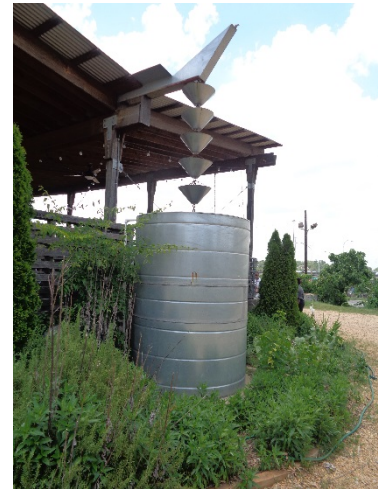
Figure 4.6.2. Example of rain chain flowing into a Cistern
