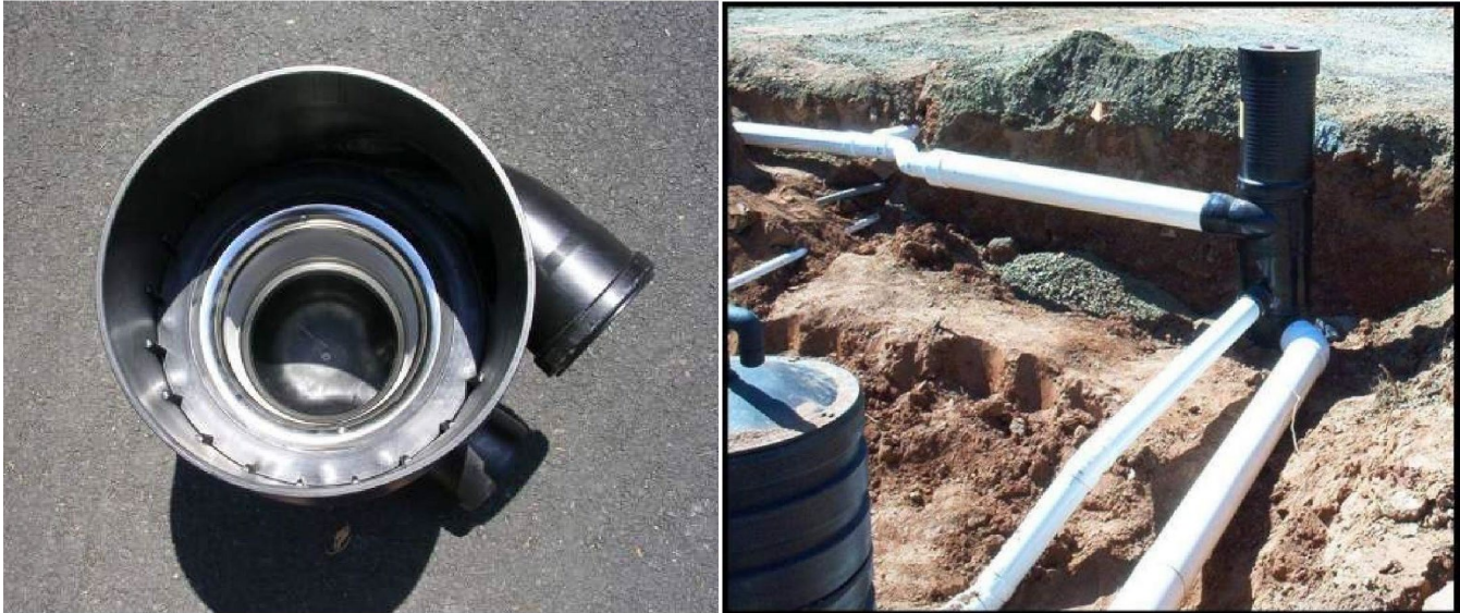
Figure 4.6.9. Interior of Vortex (left) and Installation of Vortex Filter Prior to Backfill (right)
