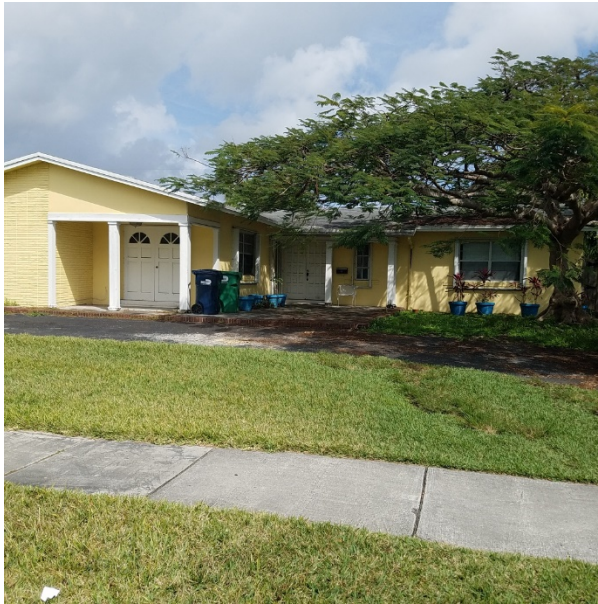
Home has partial guttering; drains next to foundation
