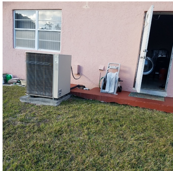
HVAC elevated to first-floor elevation
