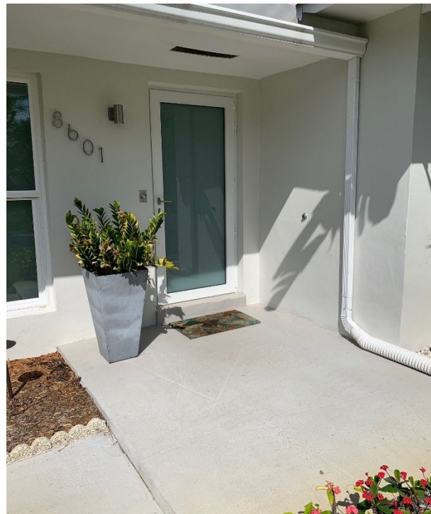
Guttering drains off front patio to garden area graded away from house
