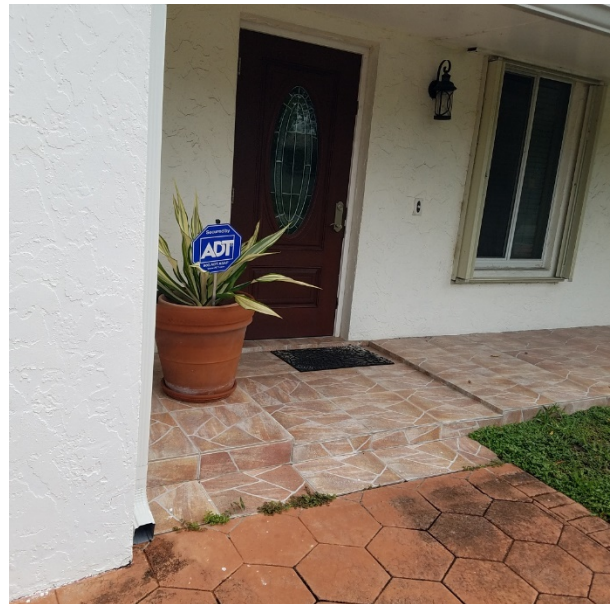
Home elevated approximately 6" above grade; guttering drains to driveway
