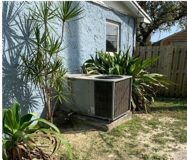
HVAC elevated less than a foot
