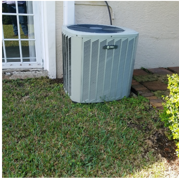
HVAC below first-floor elevation
