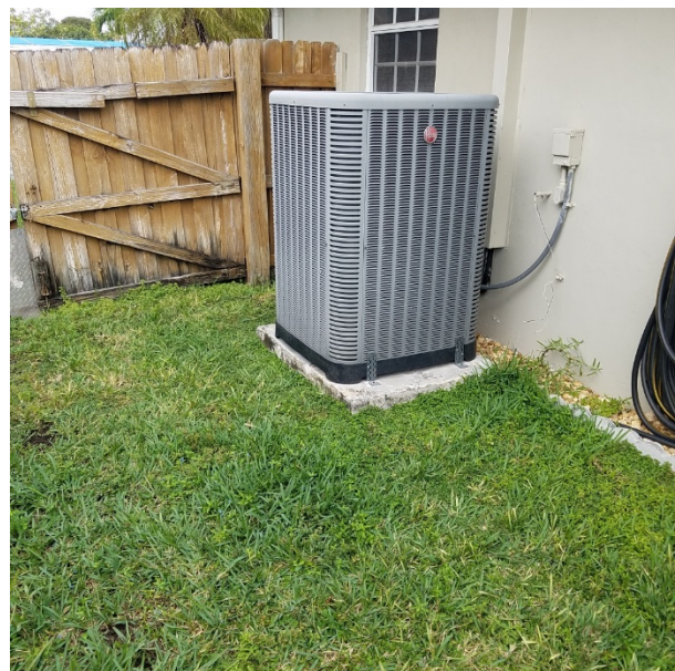
HVAC elevated approximately 4" above grade
