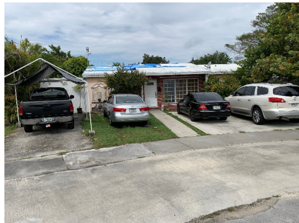
Parking pad may limit drainage away from house
