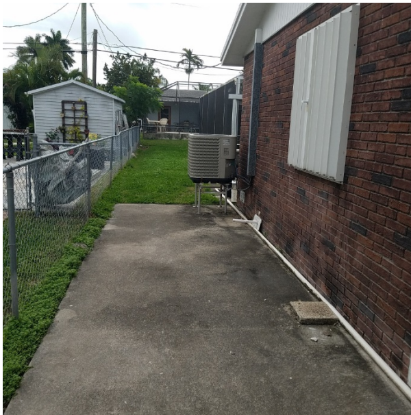
HVAC elevated above first floor elevation
