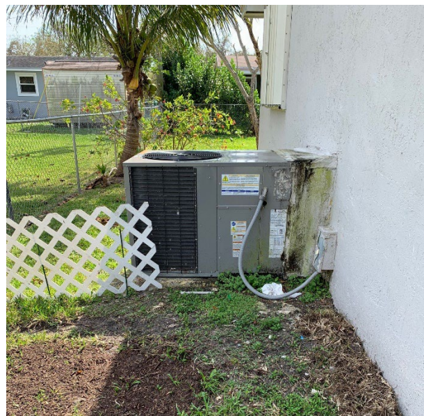
HVAC at grade
