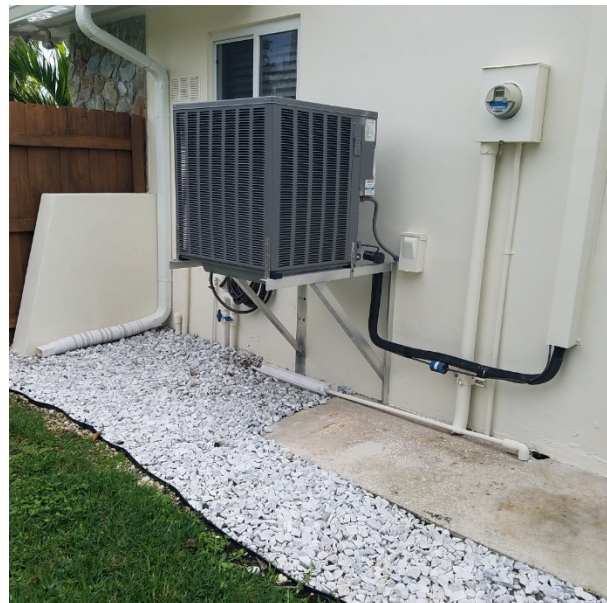
HVAC elevated and secured 3' above grade
