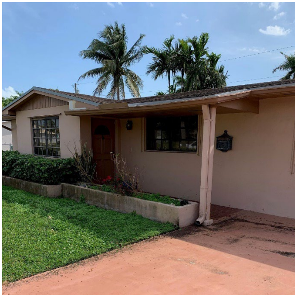
Guttering draining onto driveway
