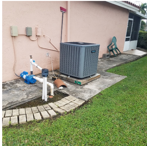
HVAC elevated above grade
