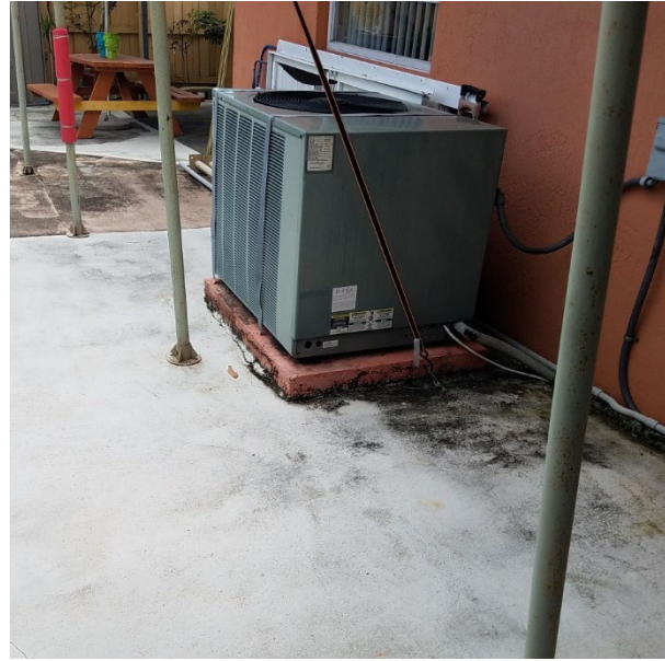
HVAC elevated approximately 4" above grade
