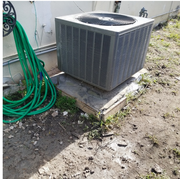
HVAC elevated approximately 6" above grade
