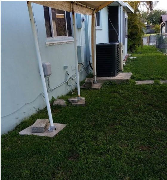
HVAC slightly elevated
