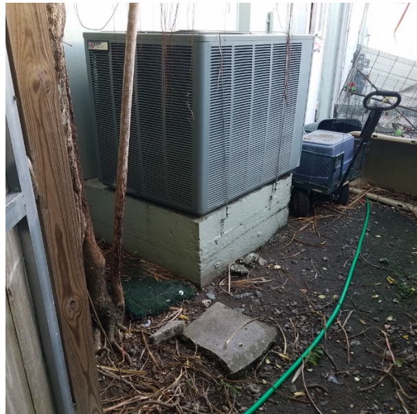
HVAC elevated nearly 2 feet above grade
