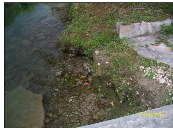
Canal Erosion on SW 194th Street
